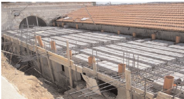
Painful reminder: On June 21, 2011, an injunction was signed by the city engineer ordering a halt to building. Due to the failure of the police to enforce the June 21, 2011 injunction work continues at the site. This photo was taken on July 1, and shows preparations to pour cement for the ceiling.
